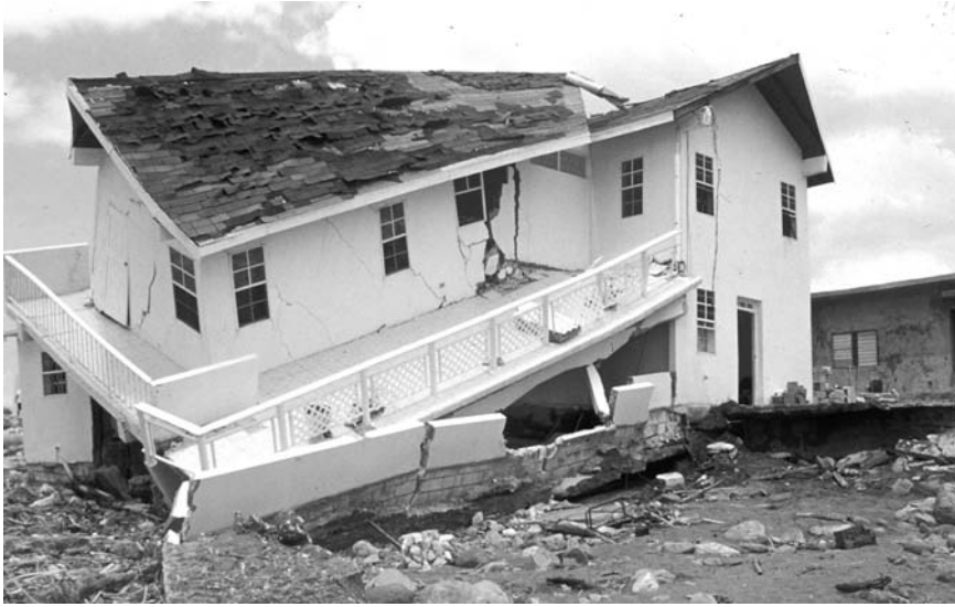
Figure 14.3 This Jamaican middle-class house was built on a vulnerable beach front location and was severely damaged by storm surge after Hurricane Ivan in 2004
